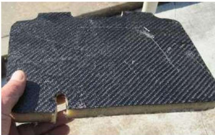
Fig. 3.53 Damage to One Face and Core (Potted Repair)
