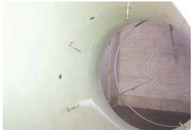
Figure 3-9. Probes within a bellmouth inlet used to measure intake temperature and pressure.
