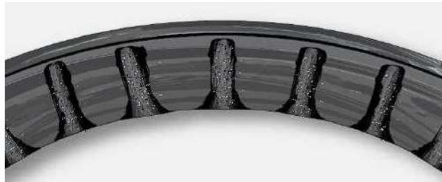
Figure 46 Staining and surface marks on the bearing cup that are grayish black streaks with the same spacing as the rollers are caused by water that has gotten into the bearing. It is the first stage of deeper corrosion that will follow.
