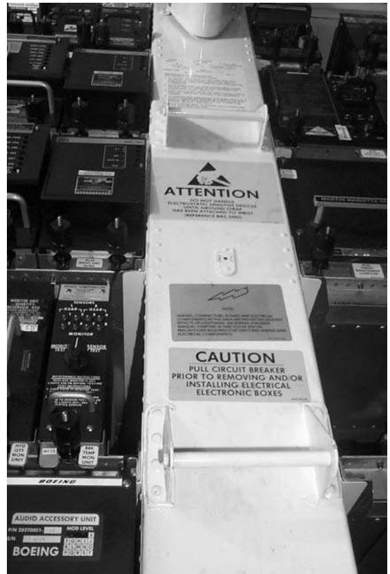
Figure 12.4 ESD warning notice (third from bottom) in the avionics bay of a Boeing 737
