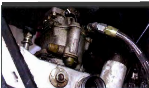
Figure 14-7. Fuel stains may indicate a leak from a worn accelerator pump seal.
