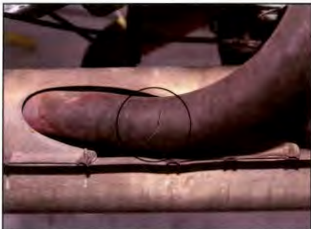
Figure 13-20. Welds in exhaust manifolds and places where exhaust gases are forced to change direction are particularly susceptible to cracks, distortion and erosion failures. Using a metal probe helps to detect deteriorated wall thickness caused by erosion. Remember to never use dissimilar metal abrasives to clean the exhaust, and do not mark components with a pencil.
