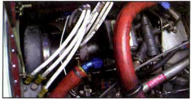
Figure 13-23. Electrical starter/generator wiring and connections must be secure to prevent abrasion, and free of corrosion or other defects.
