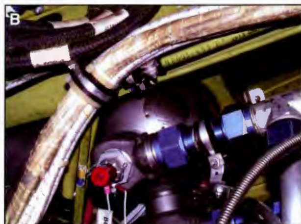
Figure 13-24. (A) Fire detection elements are inspected for condition and security of attachment. (B) Fire suppression systems are checked for weight and state of charge. Also check the expiration date on discharge cartridges or squibs.
