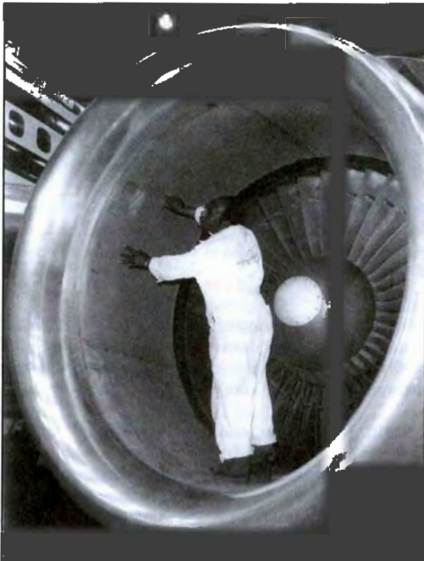
Figure 3-15. To ensure the operating efficiency of an inlet duct, you must inspect it periodically for foreign object damage and corrosion.
