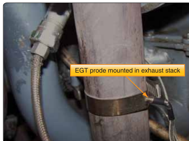
Figure 6-60. EGT probe in exhaust stack.
