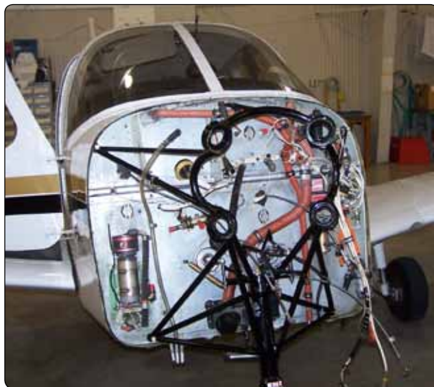
Figure 8-2. Typical firewall with components mounted on it.
