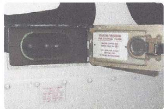
Figure 6-72. External power receptacle.
