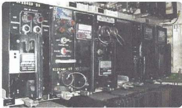
Figure 6-19. Line replaceable units in an equipment rack.
