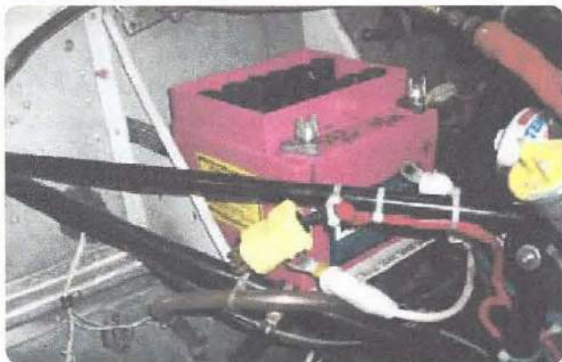
Figure 6-3. Lead acid battery installation.
