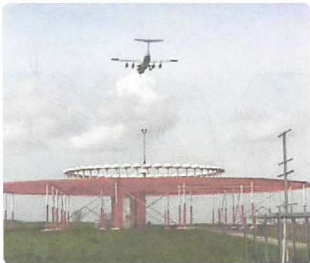
Figure 5-136. A VOR with DME ground station.
