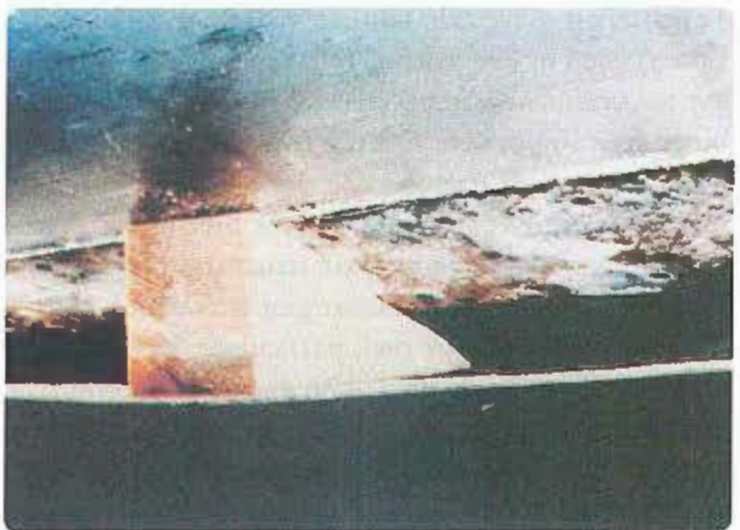
Figure 4-26. Close-up view of a corroded lap joint.
