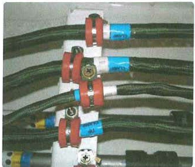
Figure 11-24. Positive separation of wire and fluid lines and wire clamps.
