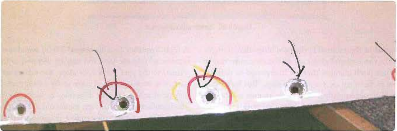
Figure 3-25. Corrosion of aluminum lightning protection mesh.
