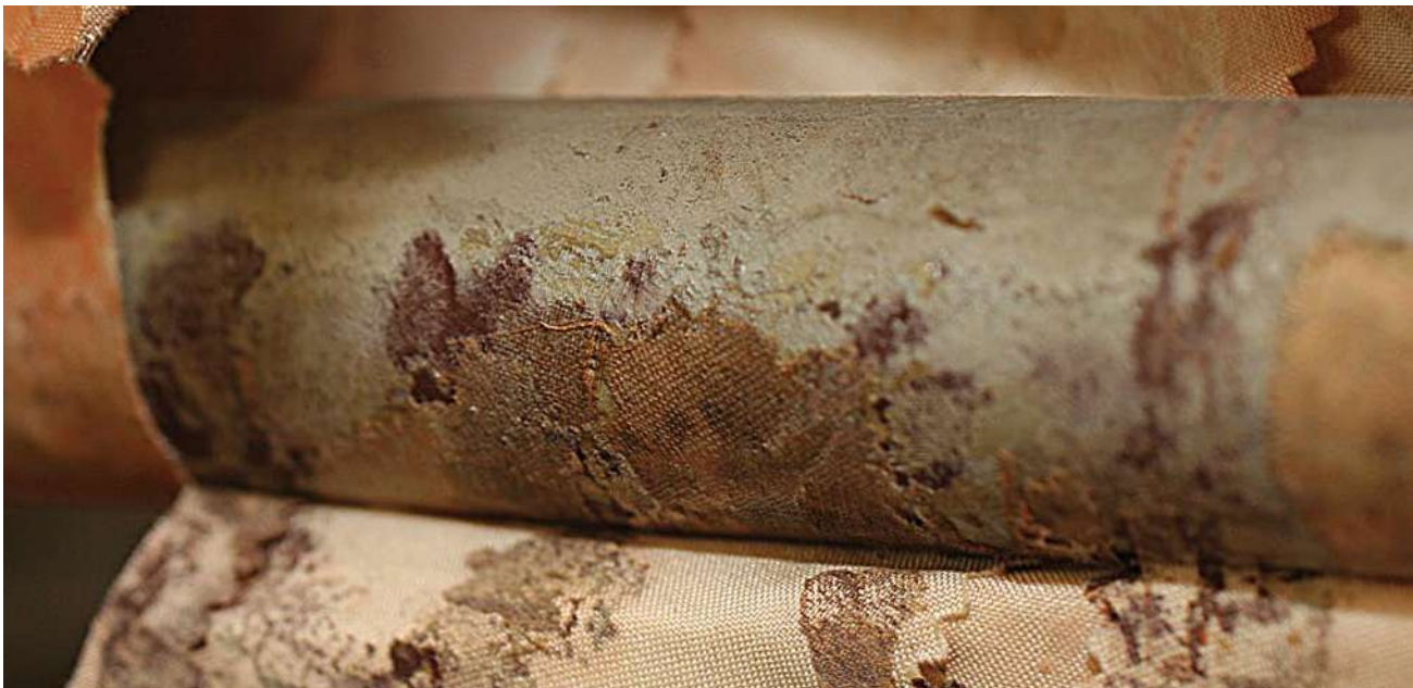
Figure 6-15. Rust on structural components.
