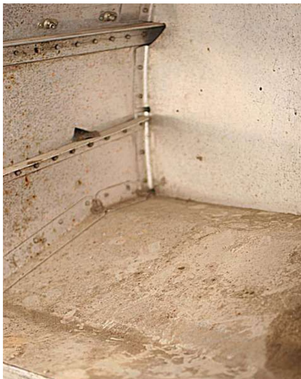
Figure 6-2. Direct chemical attack in a battery compartment.
