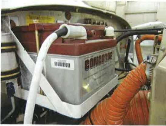
FIGURE 3-18 A 24-V lead-acid aircraft battery with self-contained battery box.
