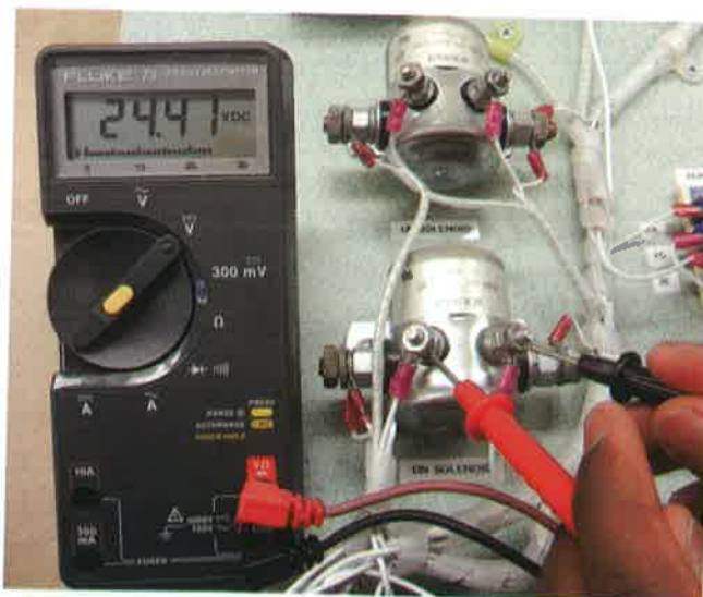
FIGURE 13-32 Digital multimeter connected to the terminals of a solenoid circuit to measure voltage.
