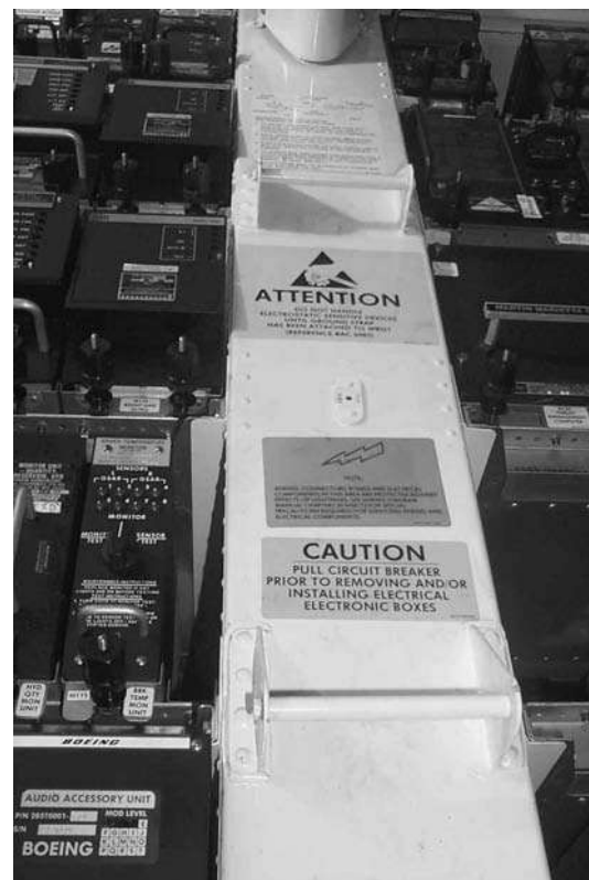
12.4 ESD warning notice (third from bottom) in the avionics bay of a Boeing 737
